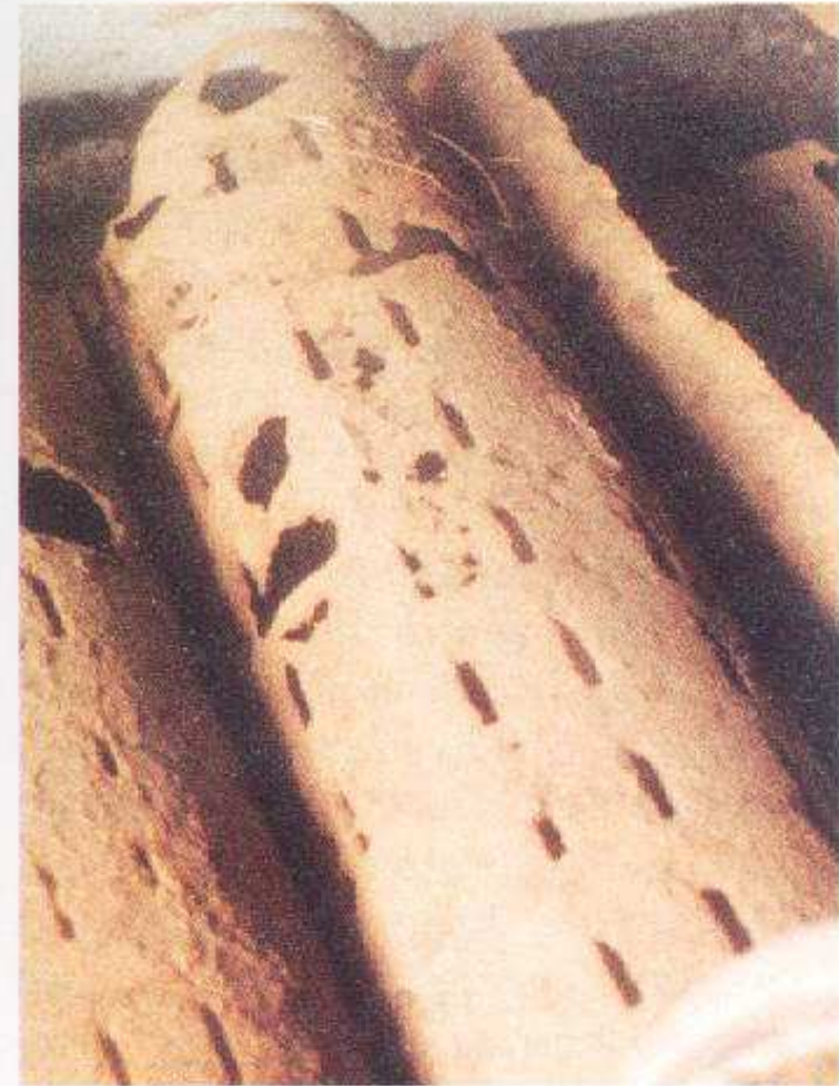
Figure 19.1. Erosion of this well screen resulted from incrustation that caused high flow velocities through the remaining open area.
